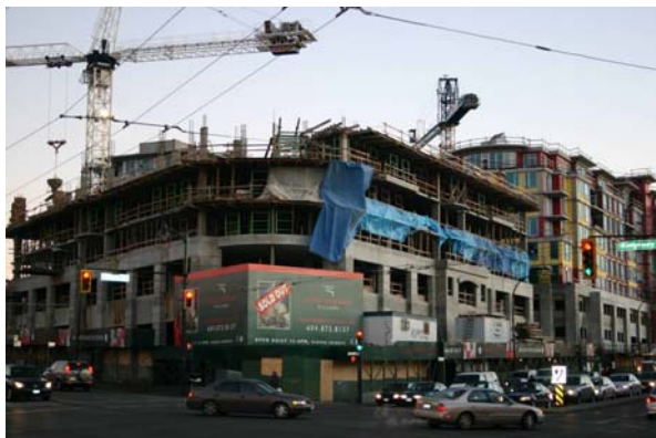
The King Edward under construction at Kingsway and Knight Street is an example of commercial use going to a mixed commercial and residential use.
